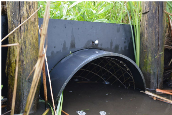
Drowning cage installed, picture by Herman Schuurman
